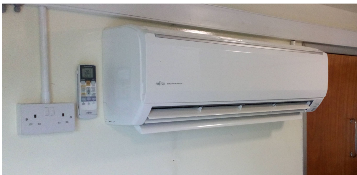
Photo 3: Wall Mounted Air Conditioning Unit at Grangemouth Zetland Park
