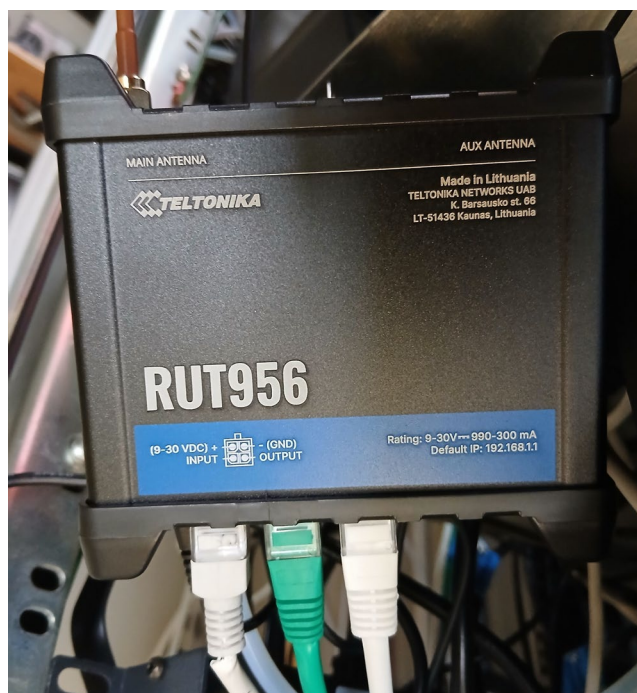
Photo 2: New 5G Data Router at the Grangemouth MC Site
